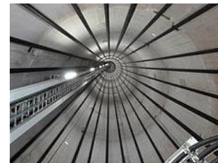
Fig 3. Inside view of a wind turbine tower, showing the tendon cables.
